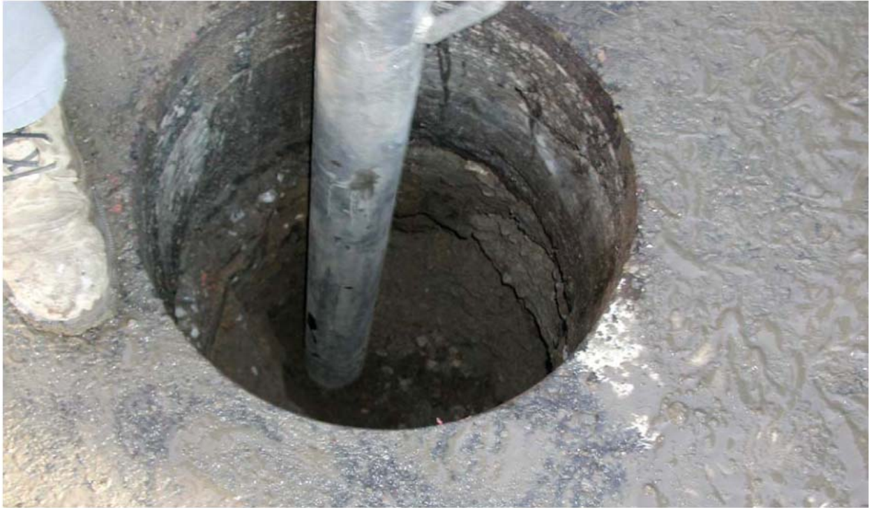
Figure 5.11. Suction pump for removing soil from the keyhole
